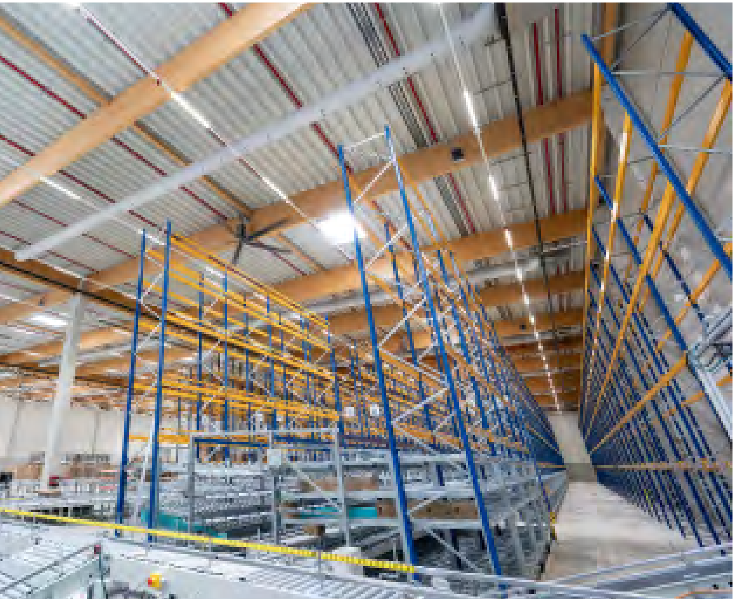
A MonsterFan circulating air for proper temperature distribution
